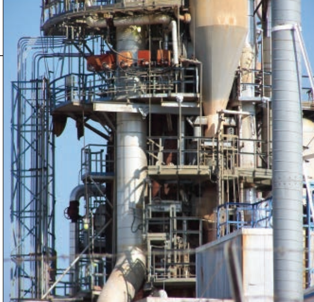
FIGURE 1. Successful completion of complex projects at petrochemical complexes, oil refineries and other CPI facilities requires close collaboration between engineering, fabrication and construction disciplines. Under an EPC contract, such collaboration must be optimized to avoid waste and errors that can result when the design attributes change after fabrication has already begun. Properly structured ERP systems can help streamline and automate the data- and project-management needs of these complex projects
