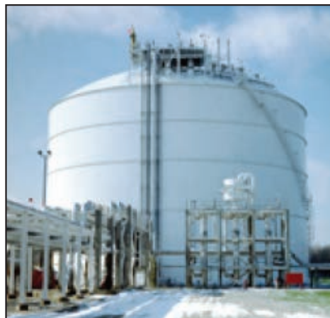
FIGURE 5. Like other process industry operations, oil & gas terminals present difficult challenges for automation and safety technology. Tank farms, storage areas, and loading/unloading operations all require fire and gas and safety systems to protect personnel, assets and the environment. The consequences of incidents at oil and gas terminals can be enormous
